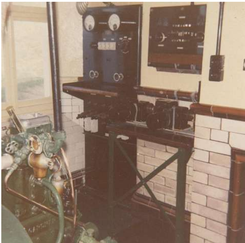
Coders and Switchboard 1974
